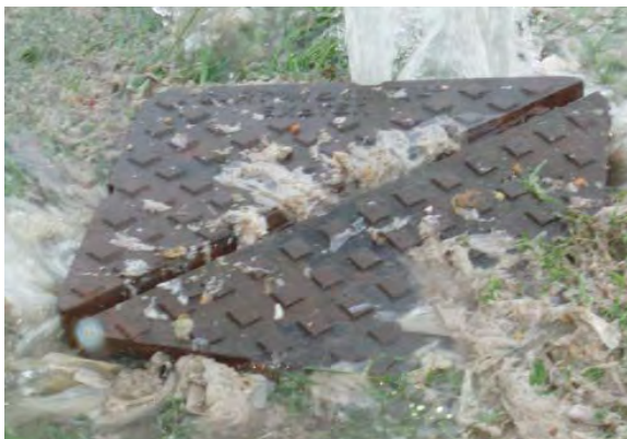
Figure 1. Sewage leaking through manhole covers. Copyright CWT.
